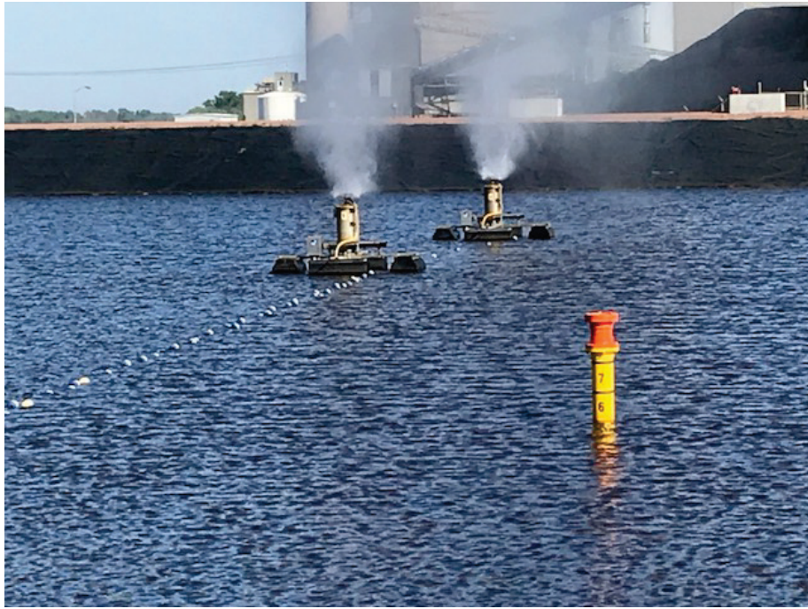
Photo 3 - 6/7/2019 – Two evaporators in operation on the Neal North Monofill leachate pond.
