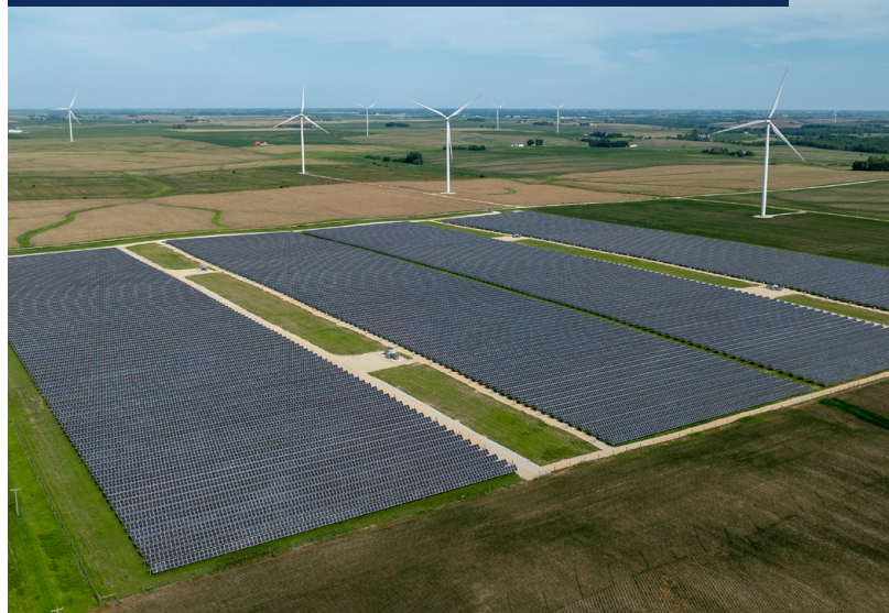
Arbor Hills Wind and Solar Projects in Stuart, Iowa.
